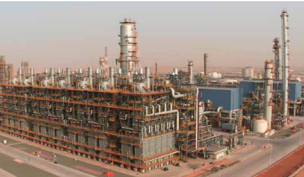
The olefin cracker at the Borouge 2 complex in Abu Dhabi is one of the world's largest plants of its kind.
