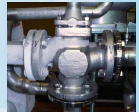
Extremely cold on the left and extremely hot at the bottom: This three-way valve must withstand enormous temperature stress.
