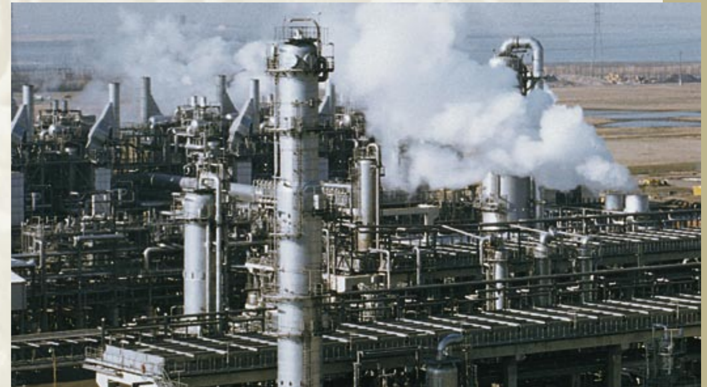
More than 1,000 SAMSON control valves, working with medium temperatures ranging between -200\text{ }^{\circ}\text{C} and +500\text{ }^{\circ}\text{C} , are installed in one of the world's largest steam crackers at Antwerp, Belgium.
