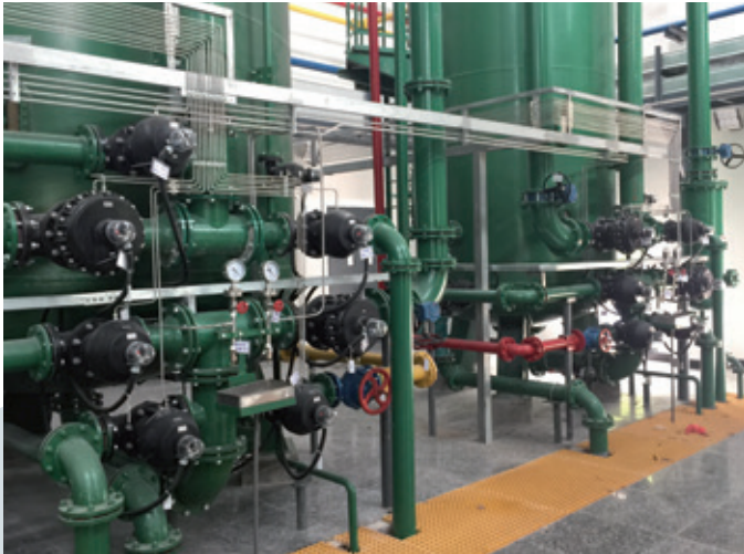
Boiled water system in coal power station
